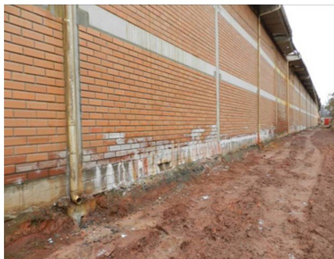
Figure 7 By-products of the reaction on the outer face of the warehouse wall.
