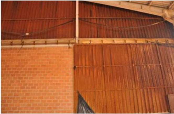
Figure 8 Metal gate (internal surface) — intense corrosion.
