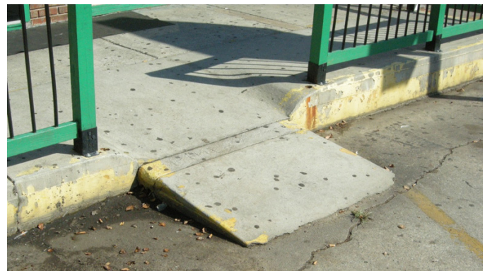
Figure 4 Combination standard and extended curb ramp. Lack of side flares on the extended portion presents a trip hazard to pedestrians approaching laterally.
