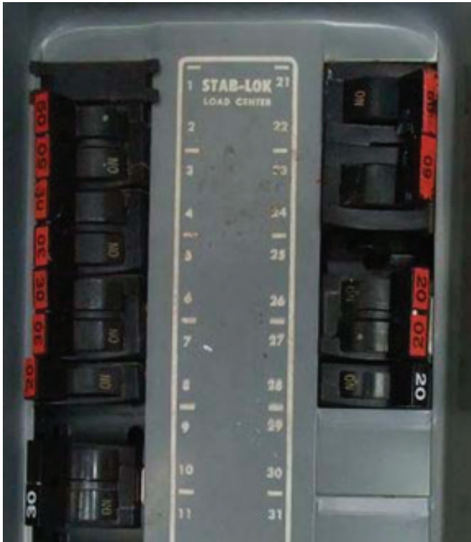
Figure 5 Federal Pacific Electric (FPE) panel.
