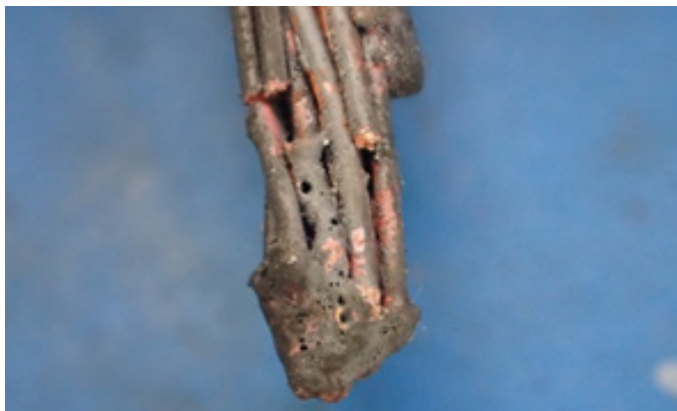
Figure 7 Arc site found on range hood wiring.
