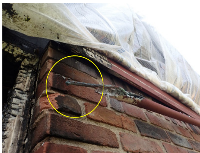
Figure 4 Arc site found on service conductors.
