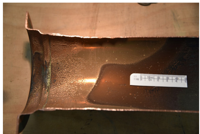
Figure 8 Copper pipe removed from service showing erosion and surface polishing where a butterfly valve was used to throttle flow rates. Flow left to right.
