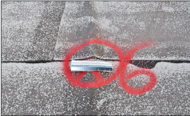
Figure 3 Area identified as wind damaged.
