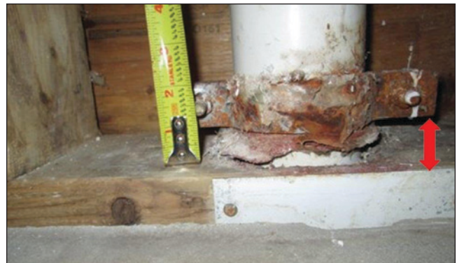
Figure 9 Riser clamp suspended above sill plate due to framing settling and pipe expansion on third floor of building.
