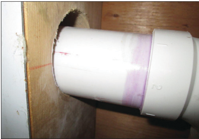
Figure 7 Horizontal piping restrained within framing.
