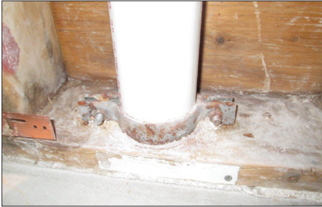
Figure 6 Vent stack pipe resting on riser clamp.
