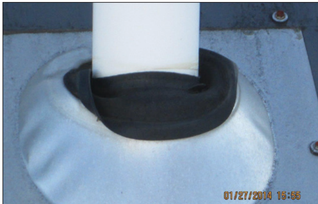
Figure 3 Damaged roof vent boot.
