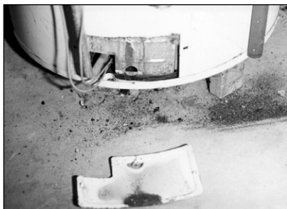
Damage from Flue Spillage and Condensation
