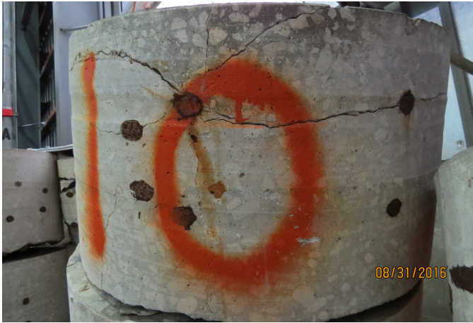
Figure 9 Concrete core with horizontal cracking.
