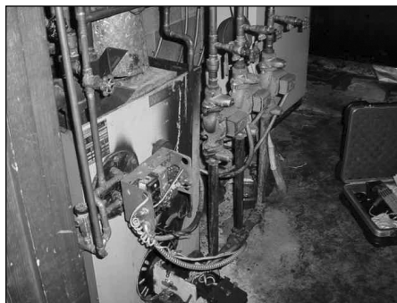
A boiler in a small room starves for combustion air.
