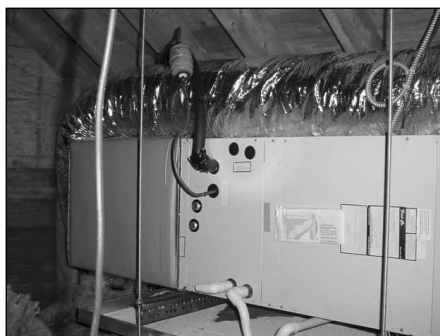
This air handler installed in a freezing attic was provided with warnings from the manufacturer as to installing it in this location.
