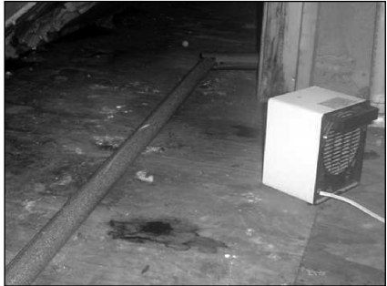
Here a domestic water pipe installed in an unheated attic is susceptible to freezing and in violation of all plumbing codes.
