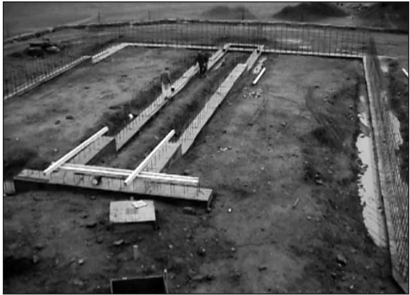
Figure 6 Water Trapped Adjacent to Footing
