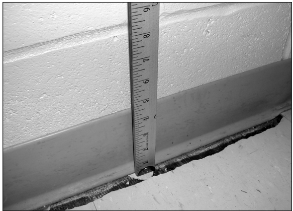
Figure 1 Differential Floor / Wall Movement
