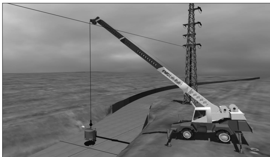
Figure 4 Crane and Power Line at Construction Site
