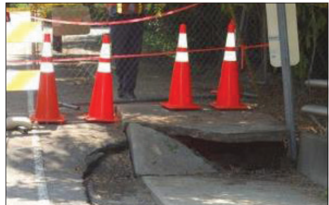
Figure 2 Settlement resulting from soil erosion at the bridge abutment.
