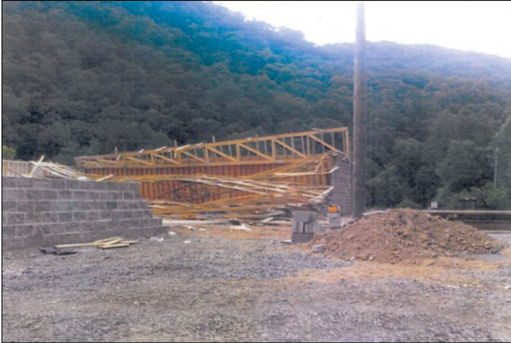
Photo 1 Front of Building After Collapse of Trusses
