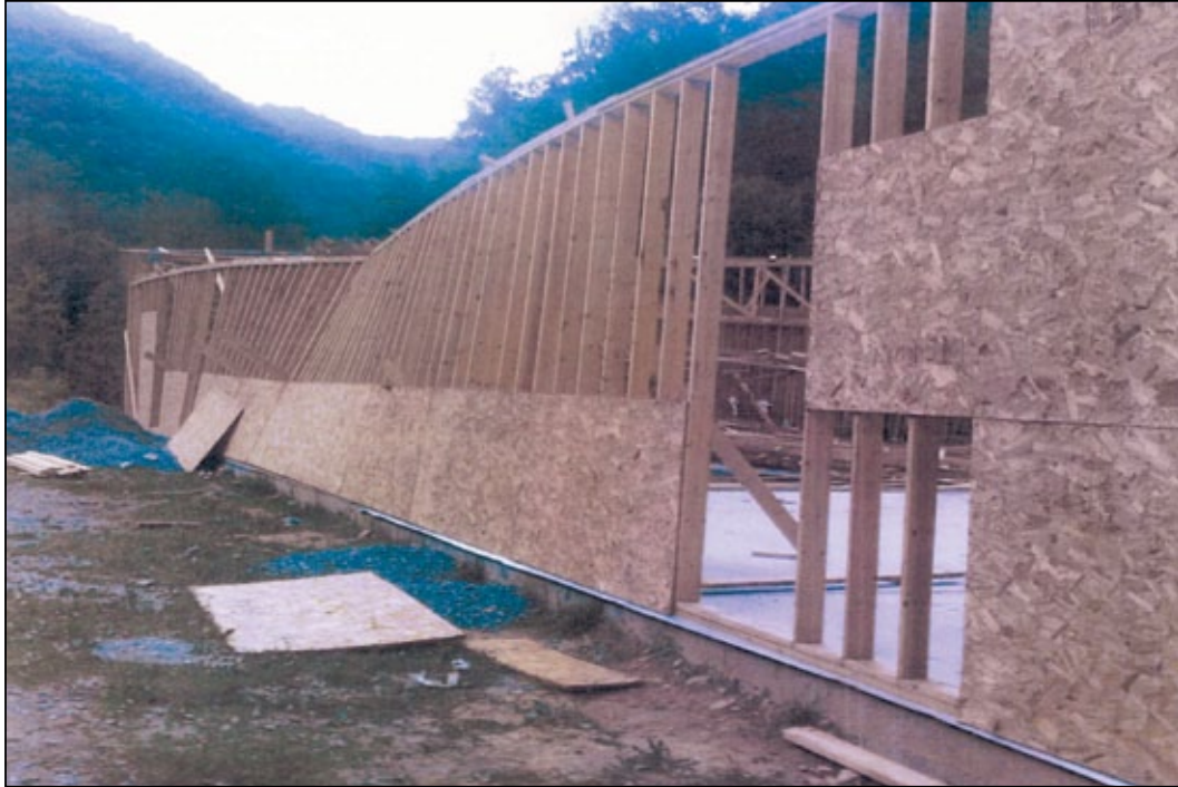
Photo 2 Back of Building After Collapse of Trusses
