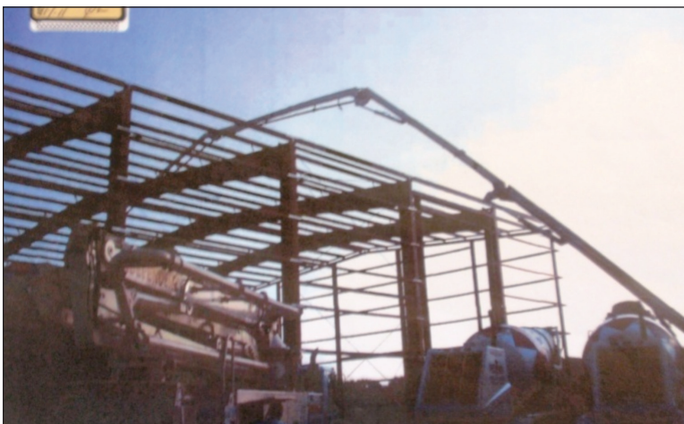
Figure 6 Concrete Pump's Boom Routed Above Roof Steel Shortening the Pump's Horizontal Reach.
