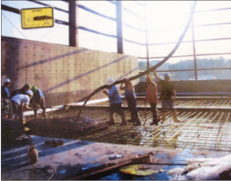
Figure 4 The Plaintiff and Co-Workers Dispensing Concrete Using the Concrete Pump's Tip Hose.
