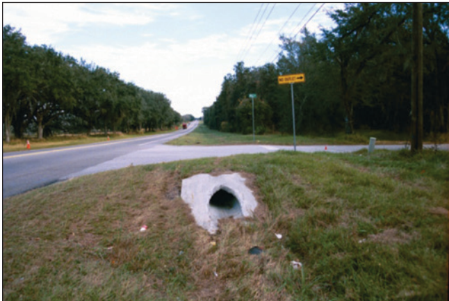
Figure 12 Accident location. SUV struck the culvert, rotated, and rolled over.
