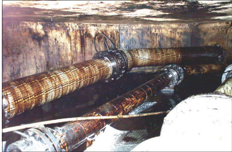
Figure 1 Concrete vault following incident, depicting fuel oil lines and flanged-end ball expansion joints
