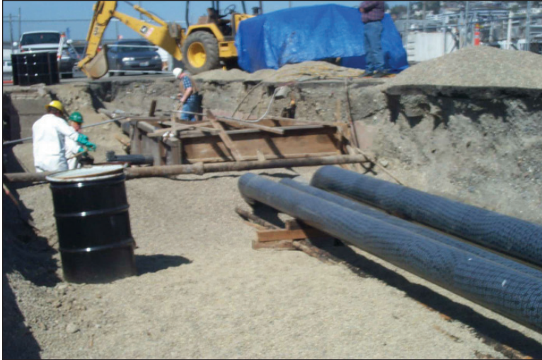
Figure 8 Typical repaired and re-wrapped piping
