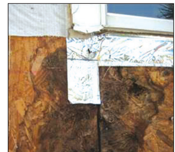
Photo 5 View of Damaged Sheathing
