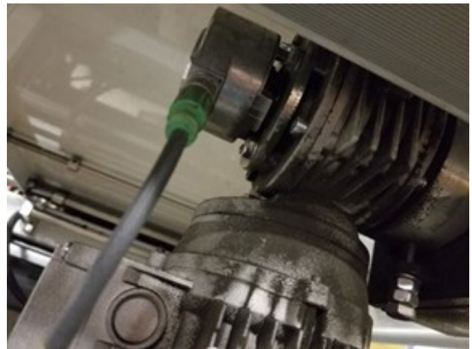
Figure 12 One of the position sensors that regularly failed shows intact cabling and shielding.
