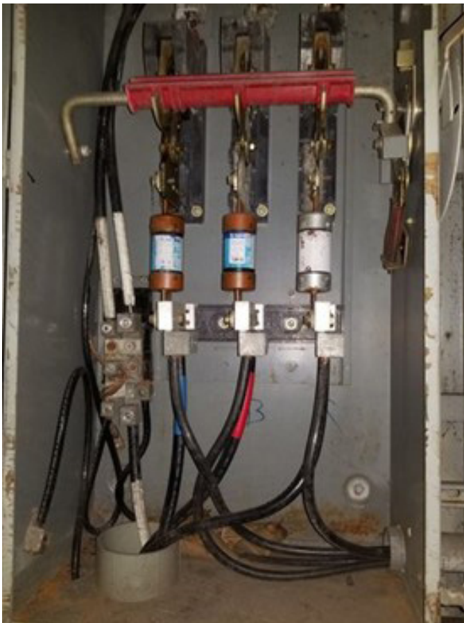
Figure 5 Panel 1, showing proper configuration of three fuses and neutral-to-ground bonding point.
