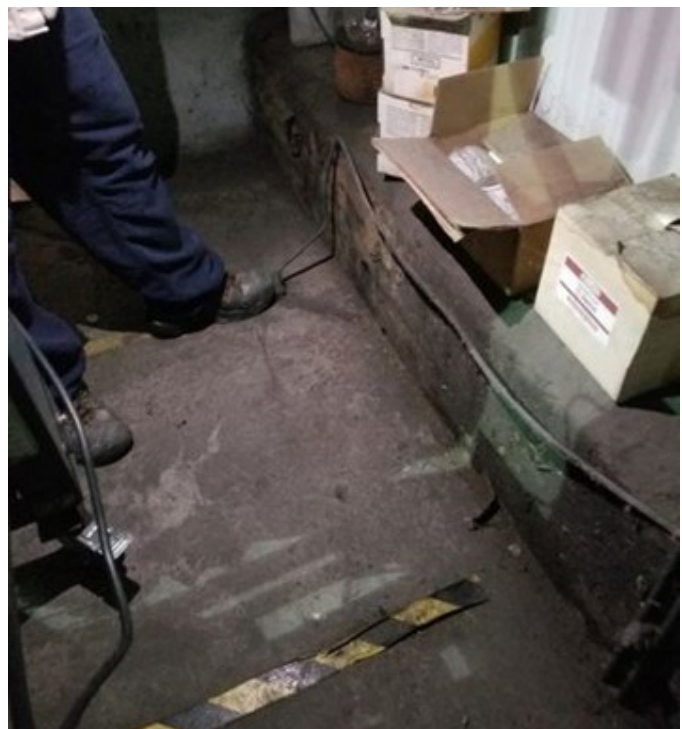
Figure 6 Service ground is established by a steel rod penetrating the foundation into the earth.
