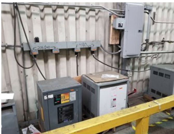
Figure 11 Panel 3 and two forklift battery chargers.
