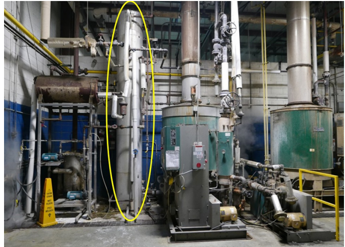
Figure 1 Exemplar SCR highlighted by the yellow circle (photograph taken by Kineticcorp).
