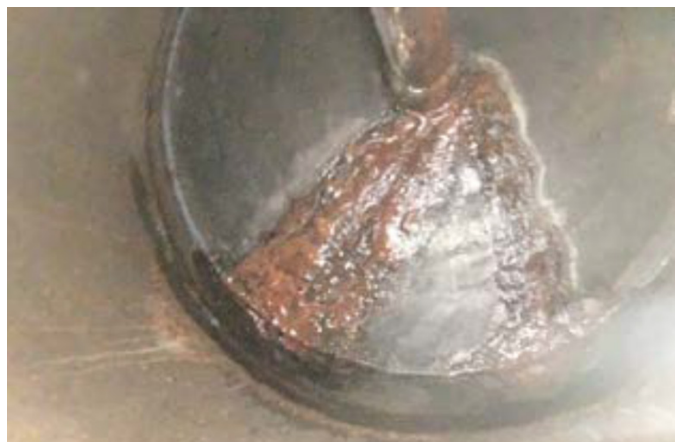
Figure 8 Picture taken by the plant engineer showing the leak from the bottom cap of the SCR.
