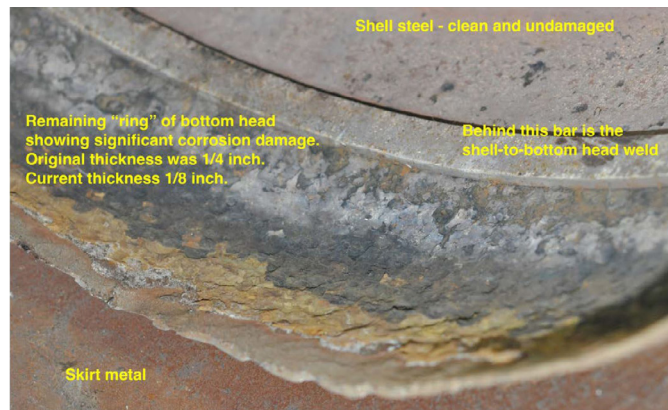
Figure 10 An image from the CSB report showing the corrosion of the 6-inch ring.
