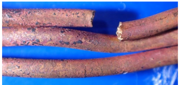
Figure 7 Example of electrical conductor mechanical damage 26 .
