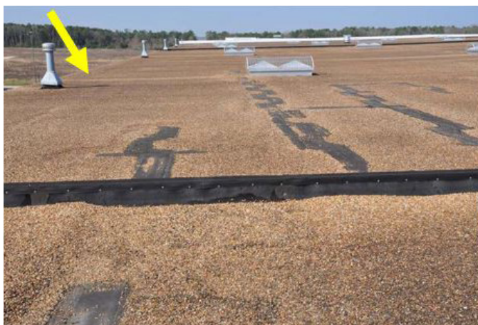
Figure 2 Fractures in the roofing membrane running parallel to the south side of the warehouse. The arrow points to the south edge of the roof.
