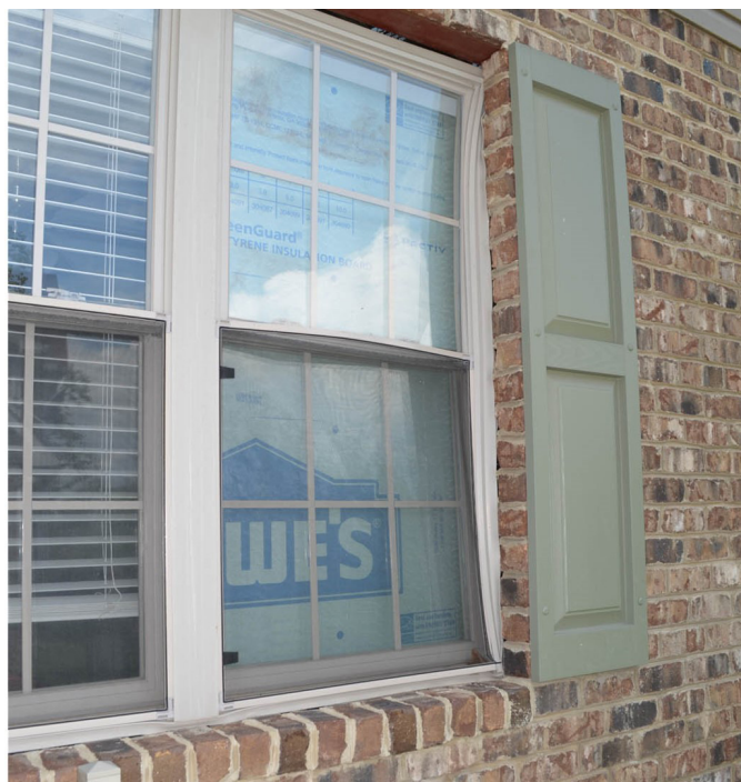
Figure 7 Right bedroom window jamb rolled beneath the right-side brick masonry veneer, buckled window screen and board insulation filling the sash space as protection against glass breakage.
