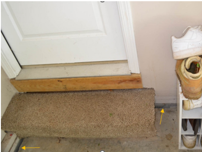
Figure 13 Garage floor separation of 1 to 1½ inches from rear and left foundation walls.
