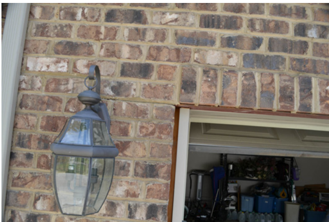
Figure 14 Front garage door jamb separation from brick masonry veneer because first level framing system was being forced rearward by connection to the front foundation wall.
