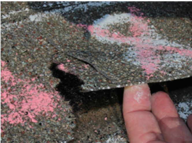
Figure 15 View of a tear along the bottom edge of an asphalt-composition shingle.
