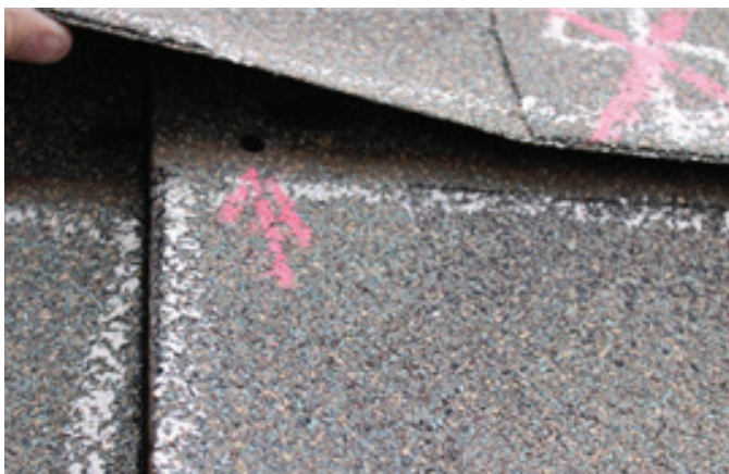
Figure 16 Shingle pulled past the nail head during the repairability assessment.
