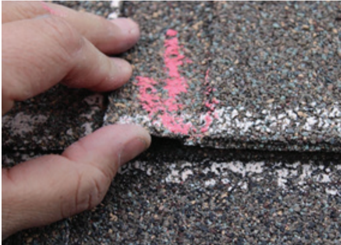
Figure 14 View of a narrow tear along the bottom edge of an asphalt-composition shingle.
