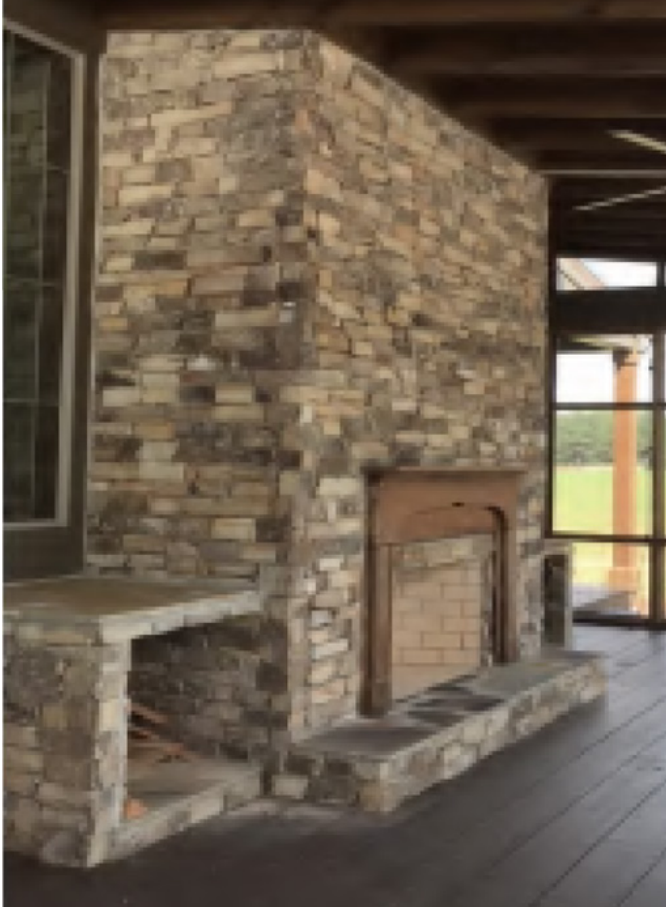
Figure 4 A view of the porch fireplace and stone veneered chase enclosure prior to the fire.
