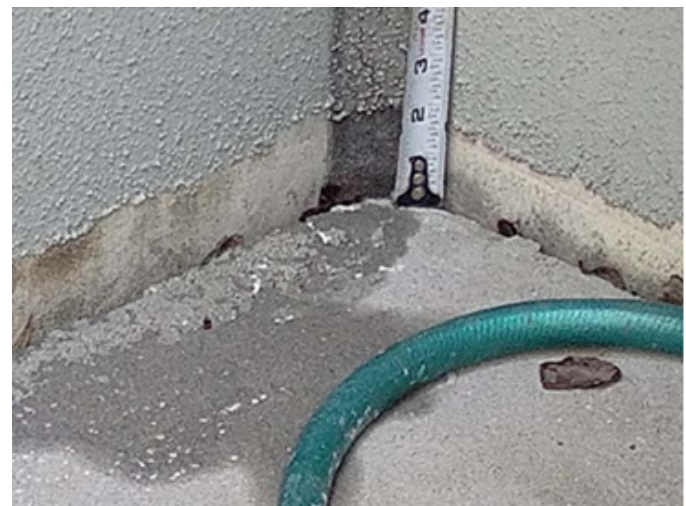
Figure 5 Up to 2 inches of slab drop in the eastern edge.
