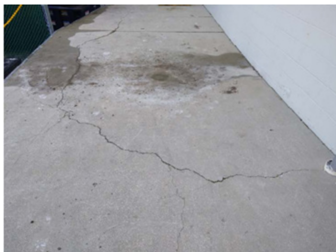
Figure 4 Up to 1/2-inch-wide crack across the slab.
