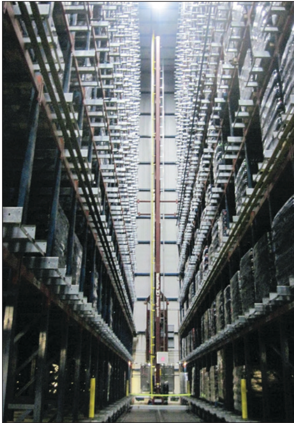
Figure 4 Storage and retrieval machine.
