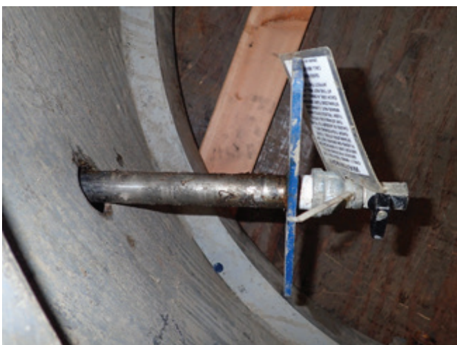
Figure 21 Test cavity bleed-off tube and valve.
