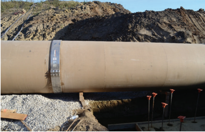
Figure 9 Pipe with external coupler.
