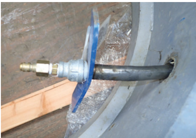
Figure 20 Test cavity fill tube.
