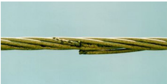
Figure 6 Neutral conductor defect.
