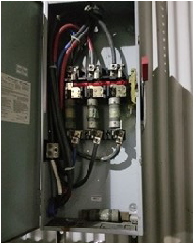
Figure 7 Internal view of Panel 2 shows neutral isolated from ground.
