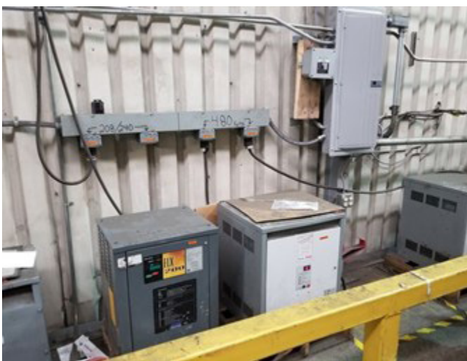
Figure 11 Panel 3 and two forklift battery chargers.
