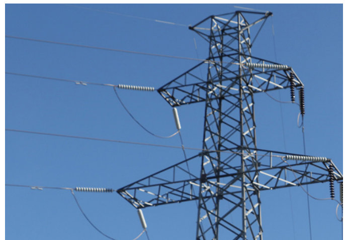
Figure 2 High-voltage transmission tower.
