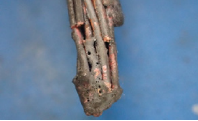
Figure 7 Arc site found on range hood wiring.
