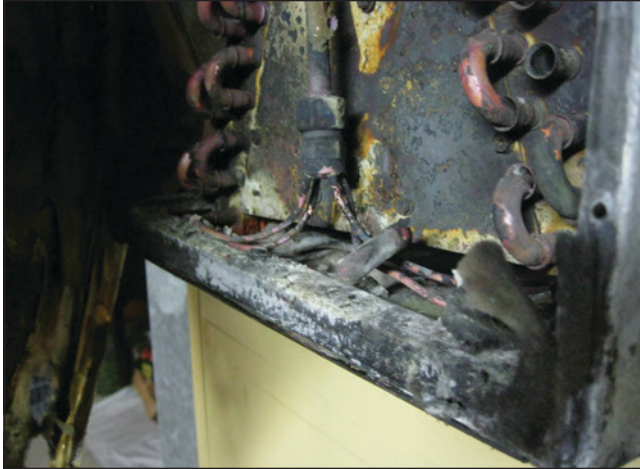
Figure 6 Heat-damaged evaporator coil and condensate pan.
