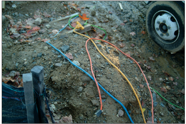
Figure 4 Various contractors' extension cords.
