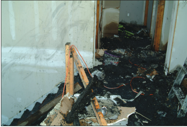
Figure 9 Extension cord leading into area of heavy damage.
