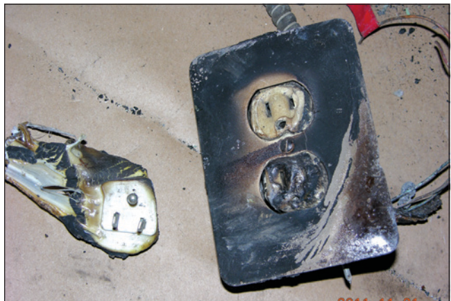
Figure 27 Plug and receptacle burned from outside in.
