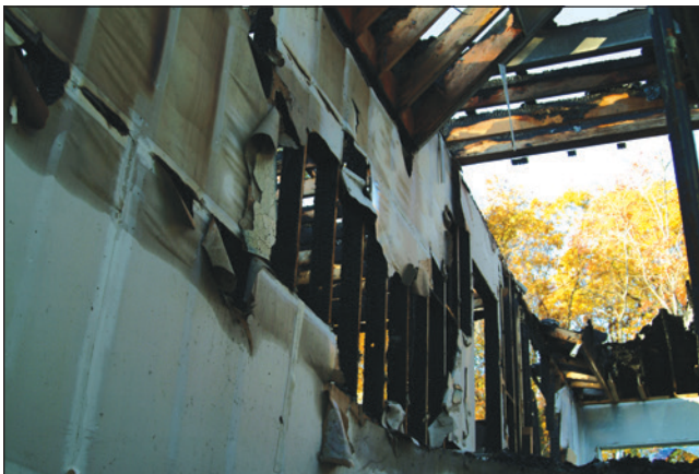
Figure 7 Fire damage from ground floor through roof.
