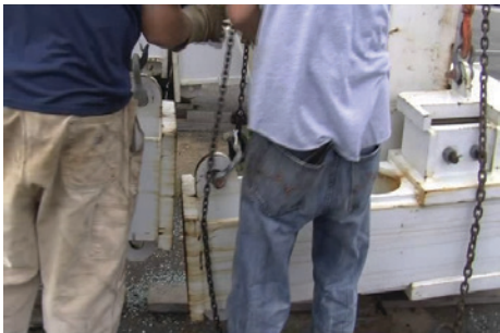
Not a clear view of two of four lever hoist required to assemble the bolted faces of collar tie.
