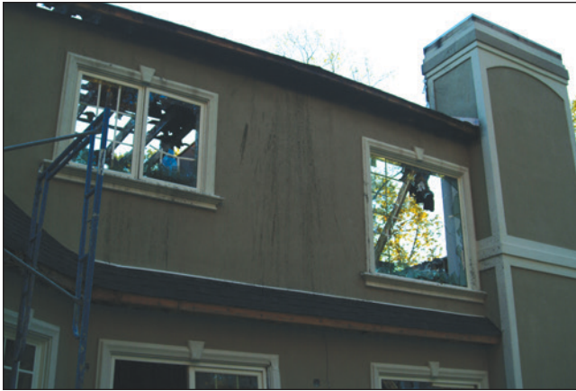
Figure 3 Interior heavily damaged.
