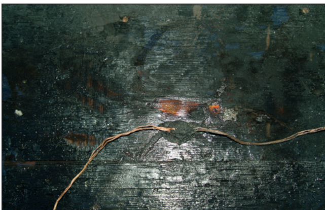
Figure 13 Extension cord (on the left), work light cord (on the right).
