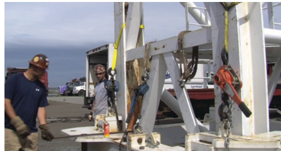
The assembled collar tie bolted out with one of two lever hoist sling combination attached at the bolted face, a manufacturer requirement.
