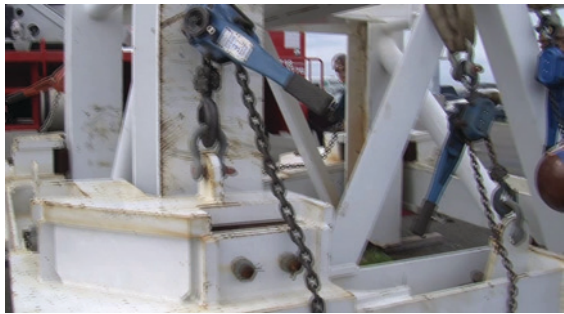
Adjusting lever hoist in place to align bolted faces of collar tie.
