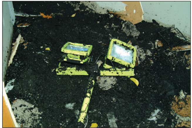
Figure 12 Work light that was plugged into the extension cord.
