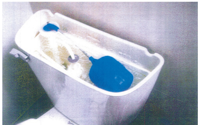
Figure 4 One of two toilet tanks with ice formation.
