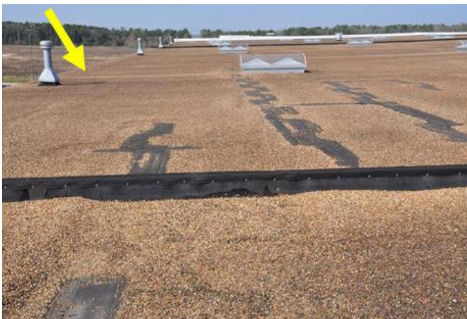
Figure 2 Fractures in the roofing membrane running parallel to the south side of the warehouse. The arrow points to the south edge of the roof.
