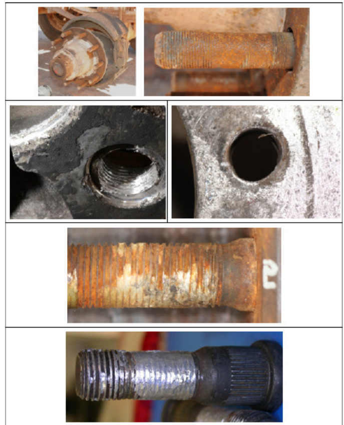
Figure 3 Examples of nut spin-off fastener failures. Top row: A left rear heavy truck axle end with missing dual wheels and brake drum. The threads of all 10 stud shanks were worn down like the one shown. Second row: wheel stud hole thread imprints from bearing on a stud and wheel stud hole elongation. Third and fourth rows: wheel metal embedment in stud threads on two left side wheel separations.
