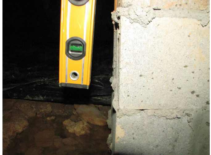
Figure 11 Right-side floor system pier measurement from plumb with active water surrounding the column.
