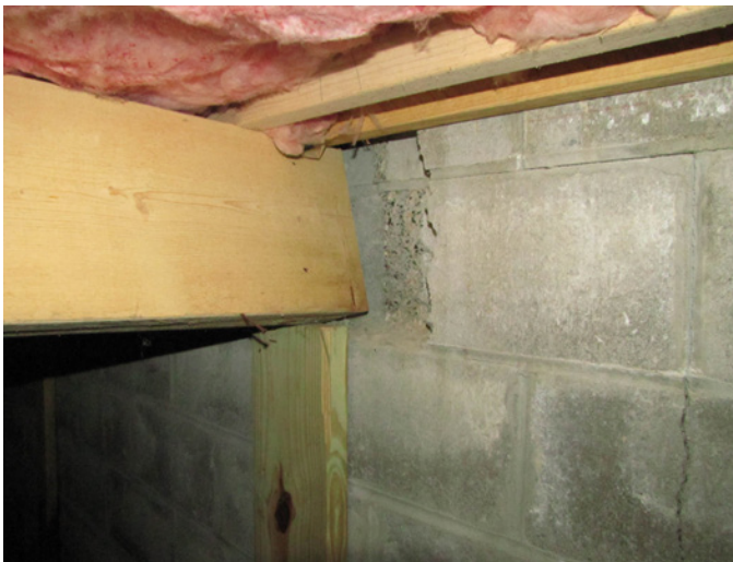
Figure 10 Right-side floor system girder displaced from its bearing seat in the front foundation wall.
