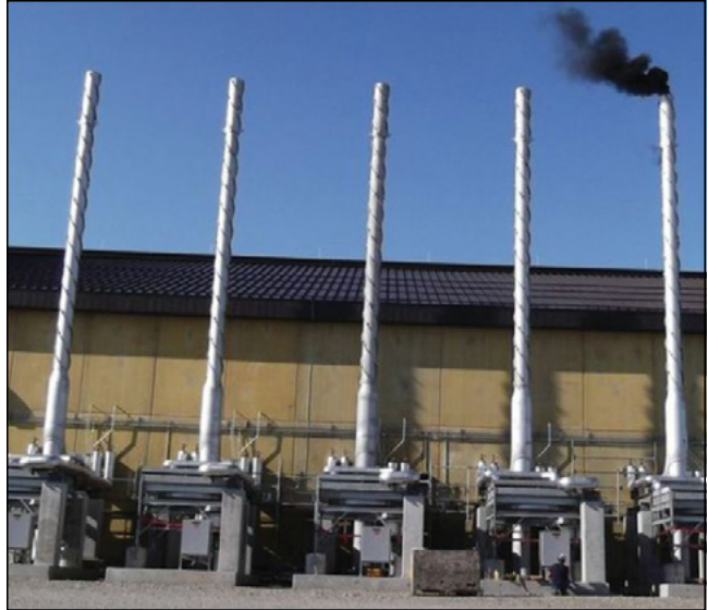
Figure 13 Strakes on stacks to prevent vibration.
