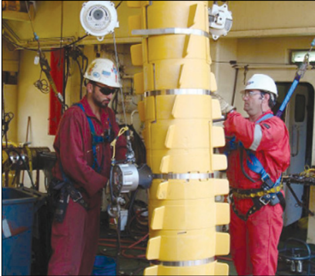
Figure 12 Strakes on subsea riser.
