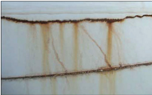
Figure 4 Crack in tower.
