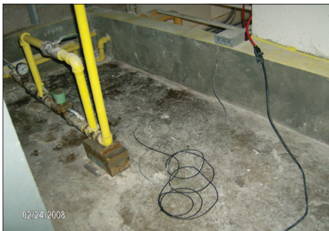
Figure 10 Fuel day tank "A" catch basin.
