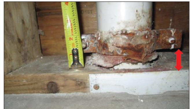
Figure 9 Riser clamp suspended above sill plate due to framing settling and pipe expansion on third floor of building.
