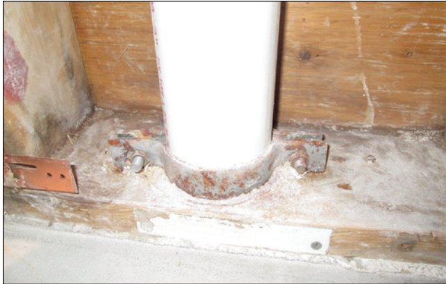
Figure 6 Vent stack pipe resting on riser clamp.
