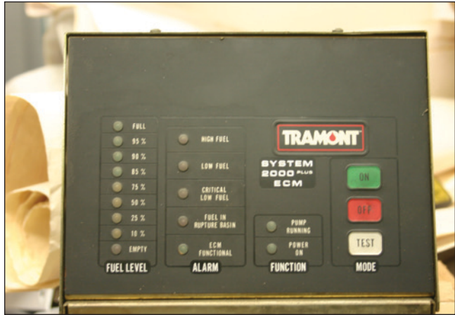
Figure 11 Fuel day tank "A" control panel (front view).
