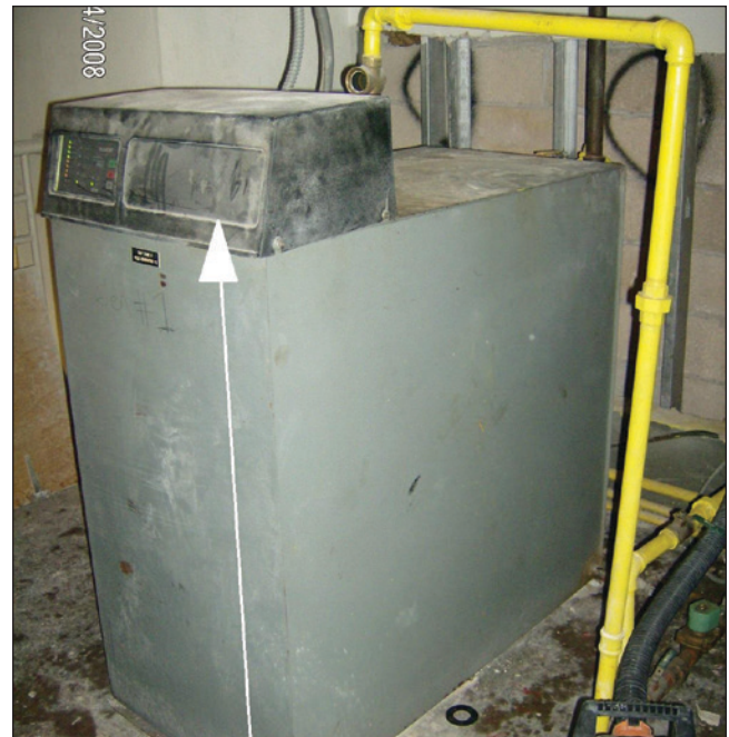
Figure 7 Fuel day tank “A” with control panel.
