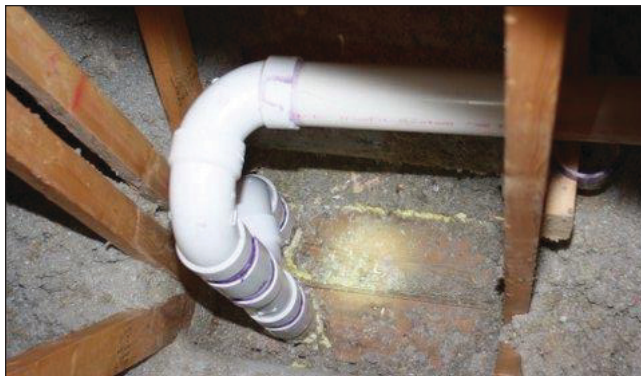
Figure 4 Vent piping entering attic space.
