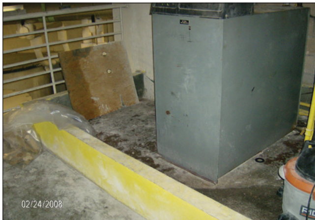
Figure 9 Fuel day tank "A" and catch basin.
