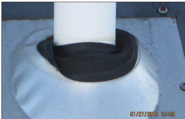
Figure 3 Damaged roof vent boot.
