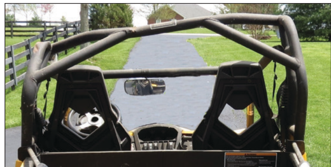
Figure 15 Case B. Rear view of failed roll cage.
