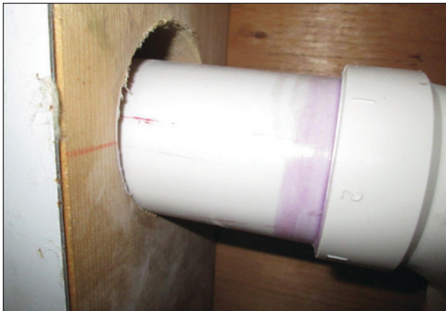
Figure 7 Horizontal piping restrained within framing.
