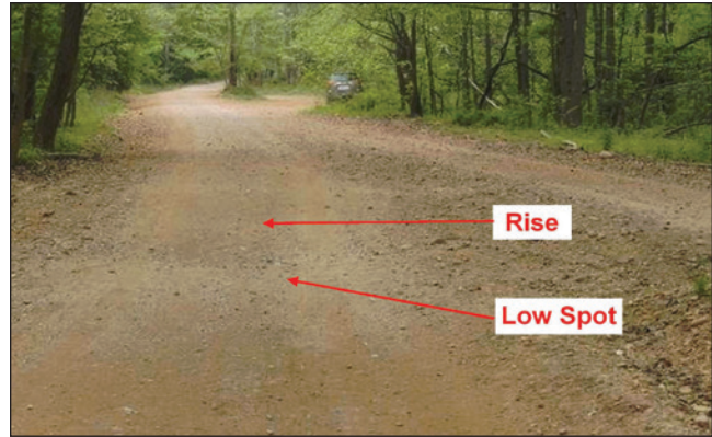
Figure 13 Case B: Accident site.
