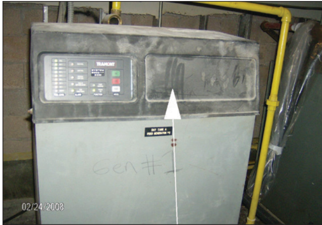
Figure 8 Fuel day tank "A" with control panel.
