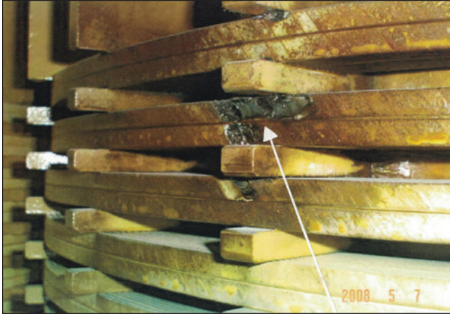
Figure 4 Transformer short circuit #1 close-up.
