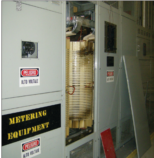
Figure 1 Transformer 13.2kV – 480/277V.
