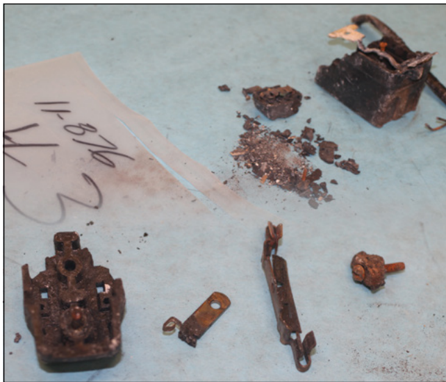
Figure 19 Evidence #3 outlet from the south wall of living room.
