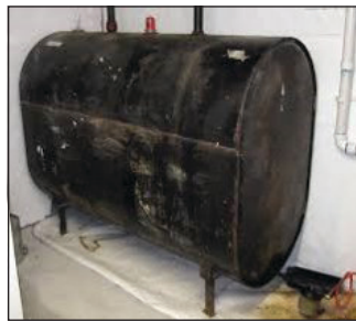
Figure 5 Typical home heating oil tank.
