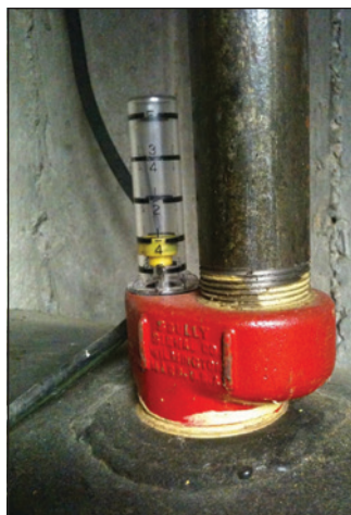
Figure 6 Heating tank gauge reading empty.
