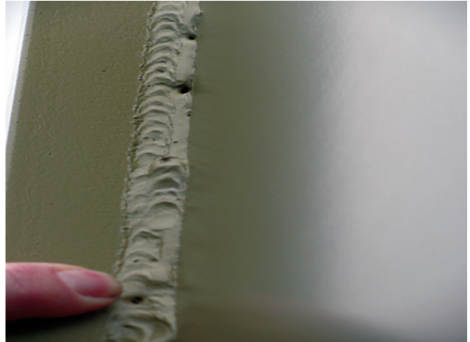
Figure 7 Typical defective weld — pores.
