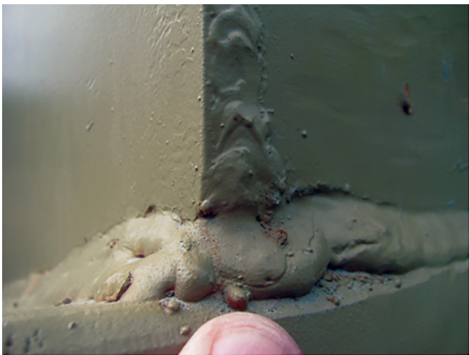
Figure 6 Typical weld defect — undercut.
