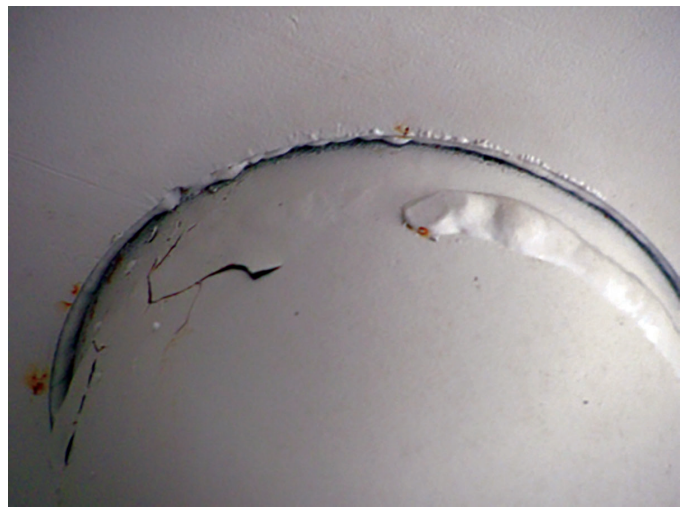
Figure 8 Typical defective weld, incomplete and non-fusion.
