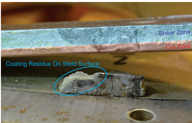
Figure 6 Failed counterweight and weld — blue area indicates shear region; the red area indicates area cut by die; the gold coating found on the weld bead surface is circled in blue.
