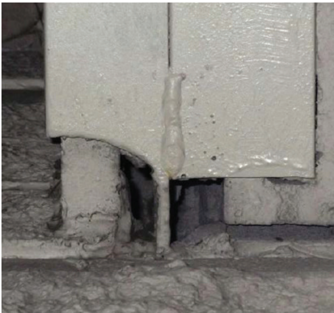
Figure 14 Incorrectly cut header.
