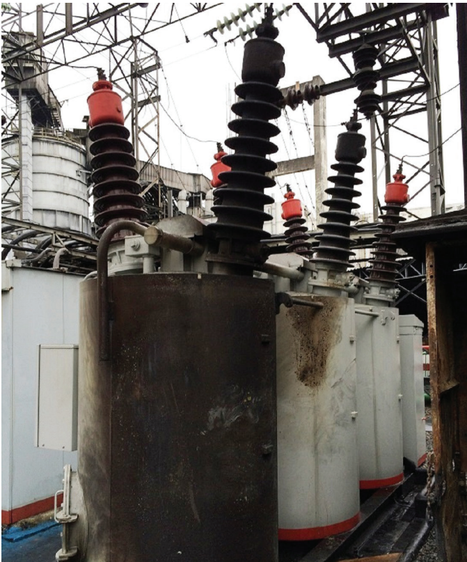
Figure 15 4.16kV circuit breaker damage.
