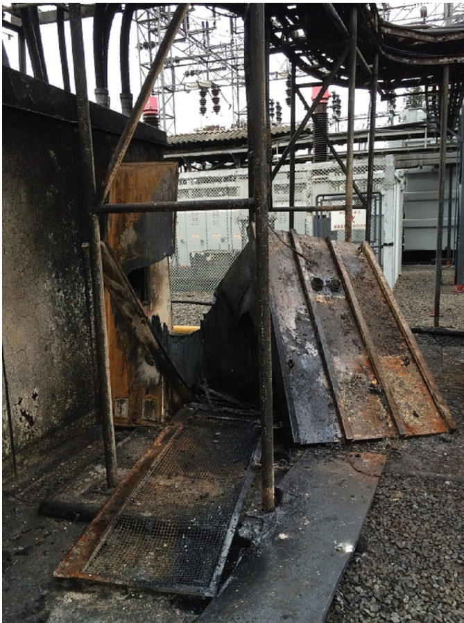
Figure 11 Cable tray fire damage.
