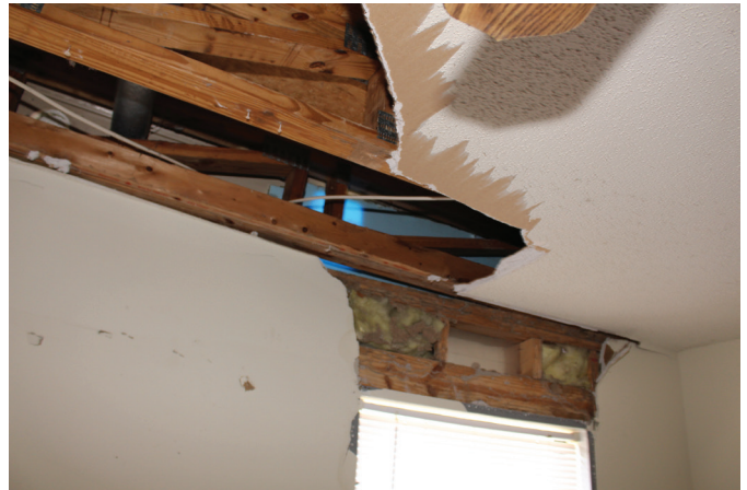
Figure 13 HVAC vent deformation and dislodgement.
