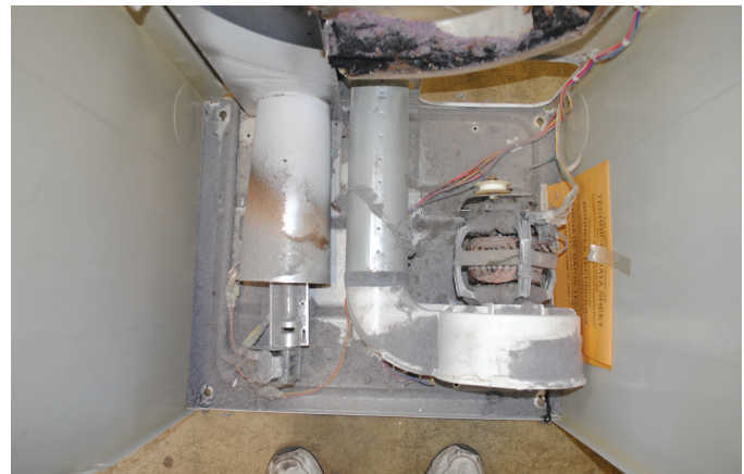
Figure 19 Accumulated lint in base of dryer.
