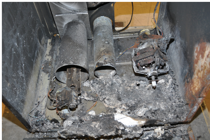
Figure 31 Base of dryer showing mostly consumed combustible plastic components.
