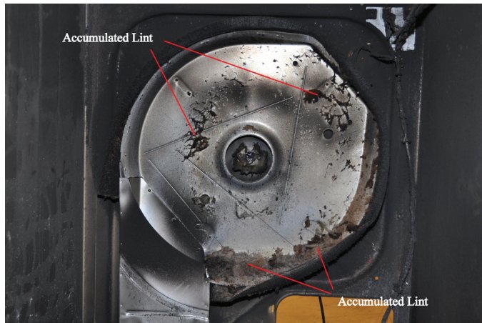
Figure 29 Heater pan of dryer showing accumulated lint.
