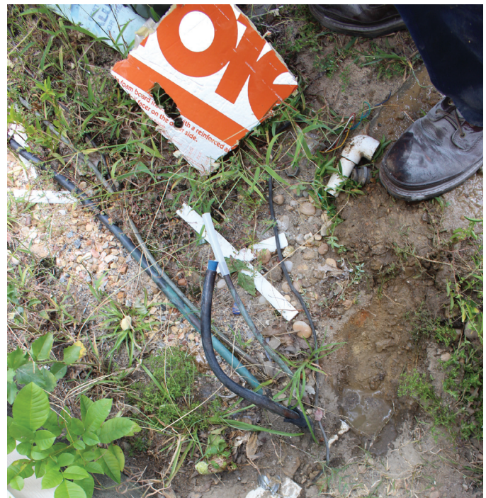
Figure 5 Excavated PVC conduit — the refrigerant pipe set from the outdoor unit entered the buried PVC conduit.
