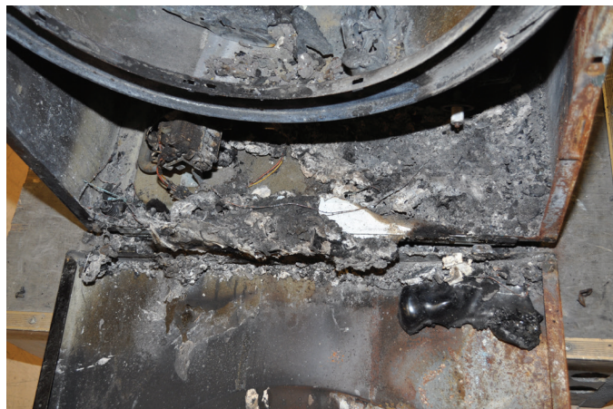
Figure 30 Base of dryer showing mostly consumed combustible plastic components.
