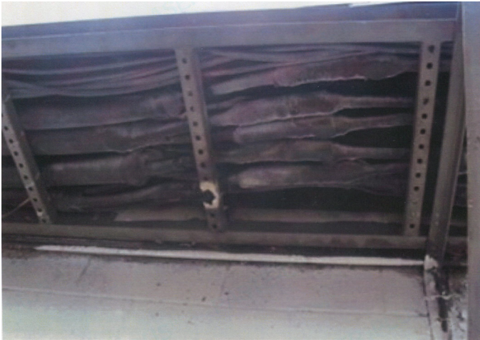
Figure 6 Capacitor bank cable splices.
