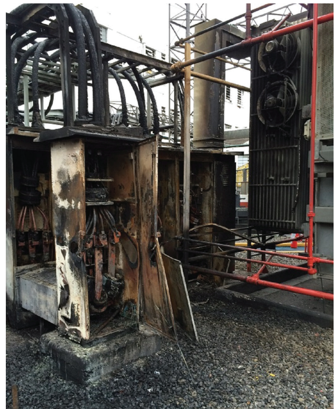
Figure 13 4.16kV switchgear damage.
