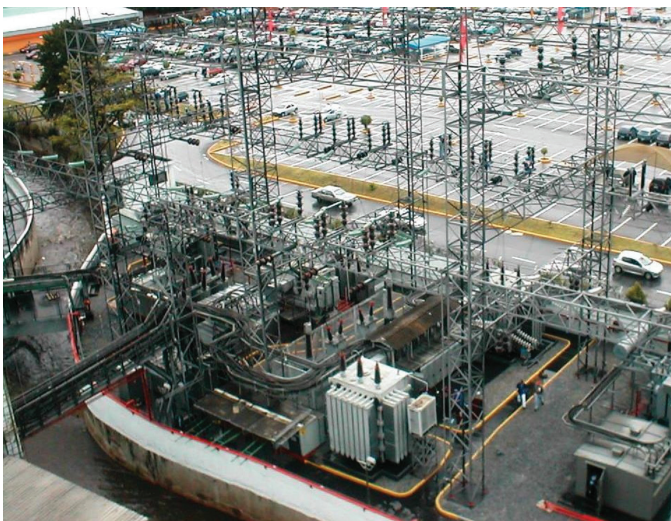
Figure 2 Partial view of substation (north view).
