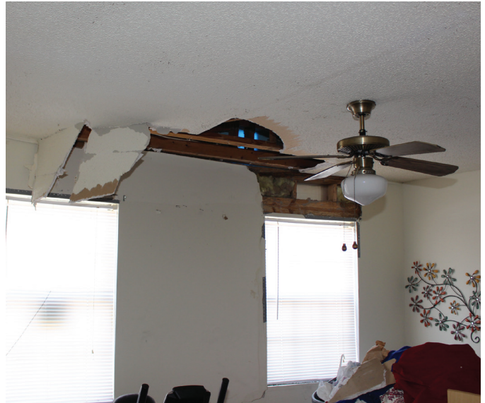
Figure 12 Interior and exterior walls separated from ceiling structures — windows intact.
