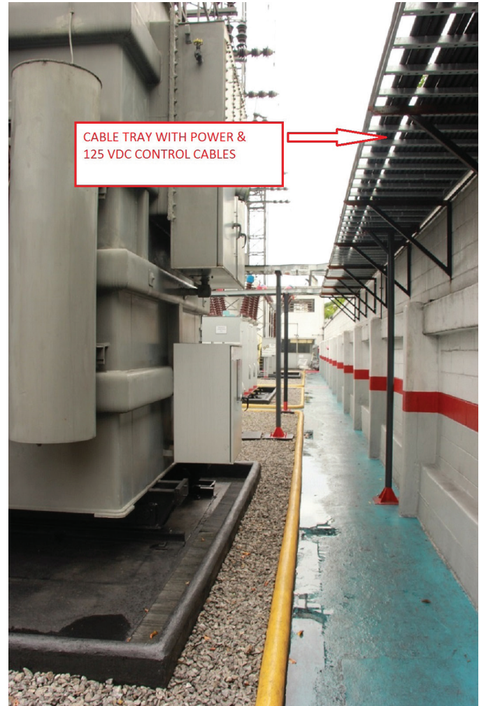
Figure 5 Cable tray for capacitor bank cables.
