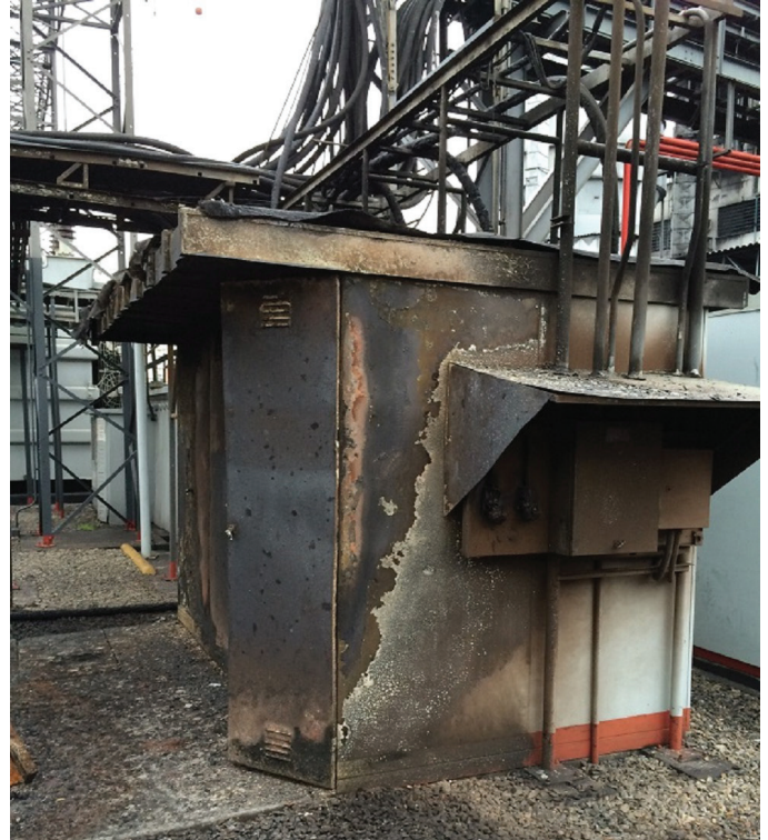
Figure 12 4.16kV switchgear fire damage.
