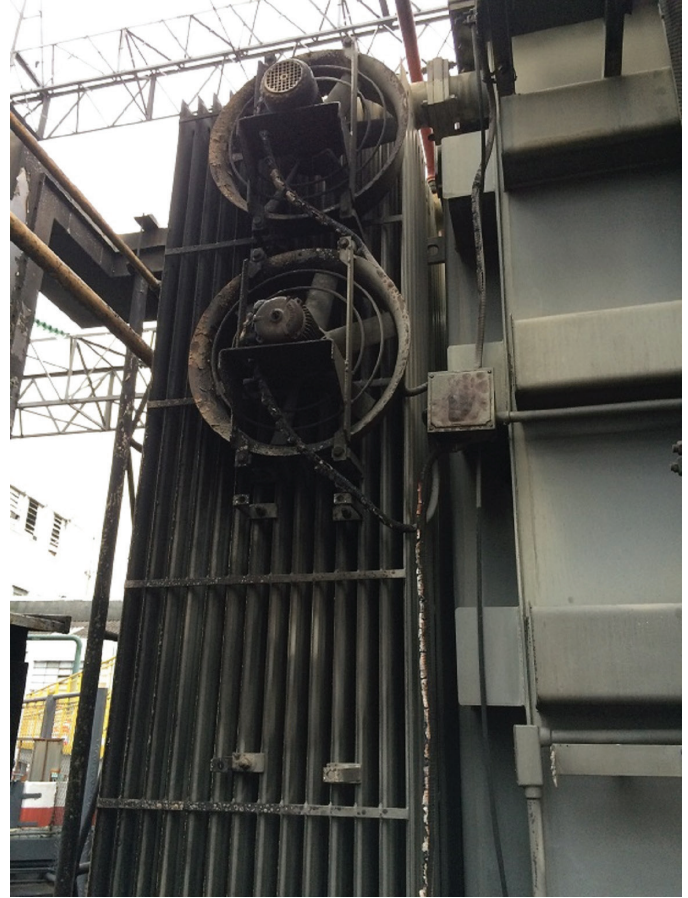
Figure 16 88kV - 4.16kV transformer damage.
