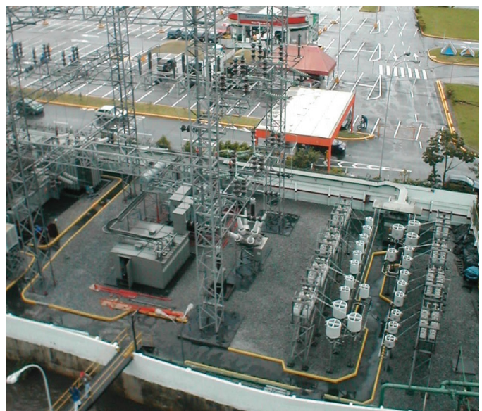
Figure 3 Partial view of substation (south view).
