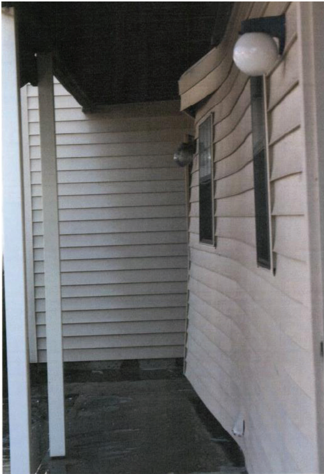
Figure 10 Exterior walls dislodged.
