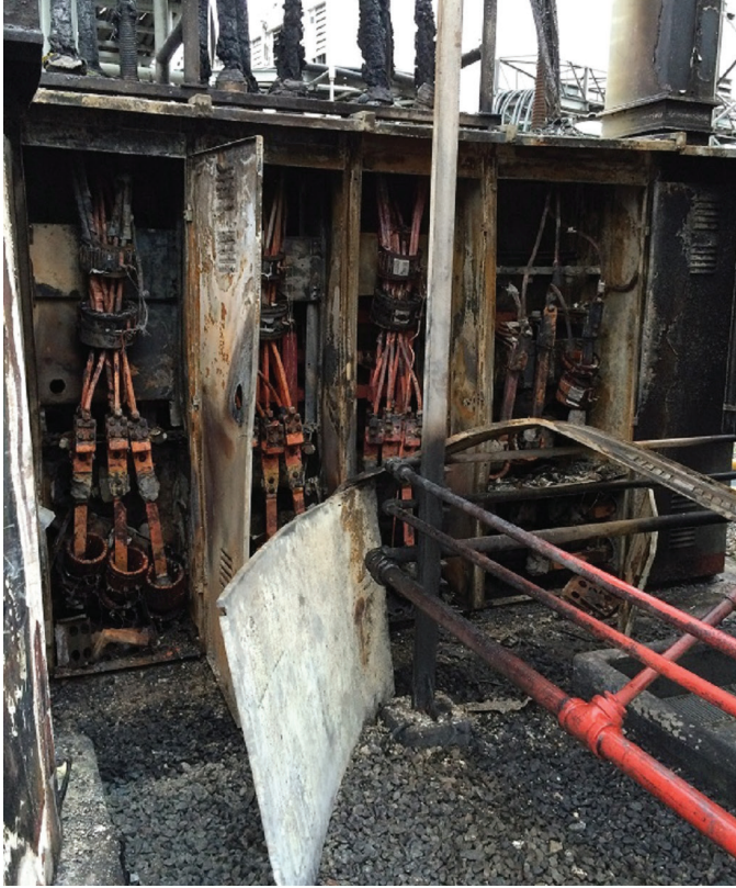
Figure 14 4.16kV switchgear fire damage.
