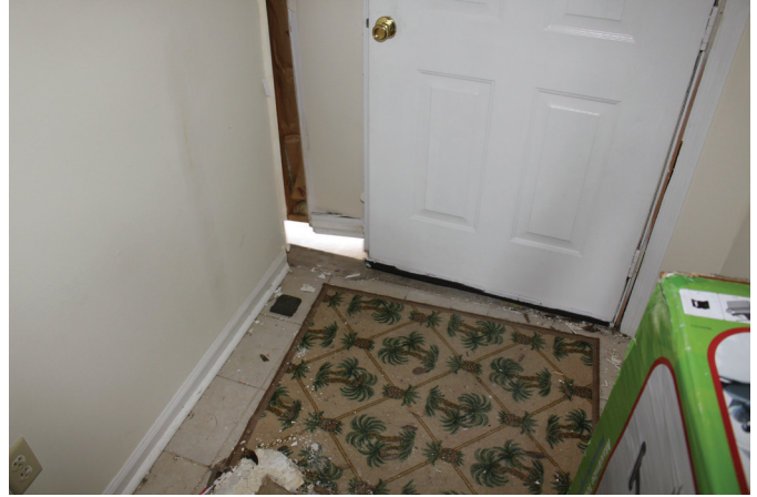
Figure 11 Exterior walls dislodged.
