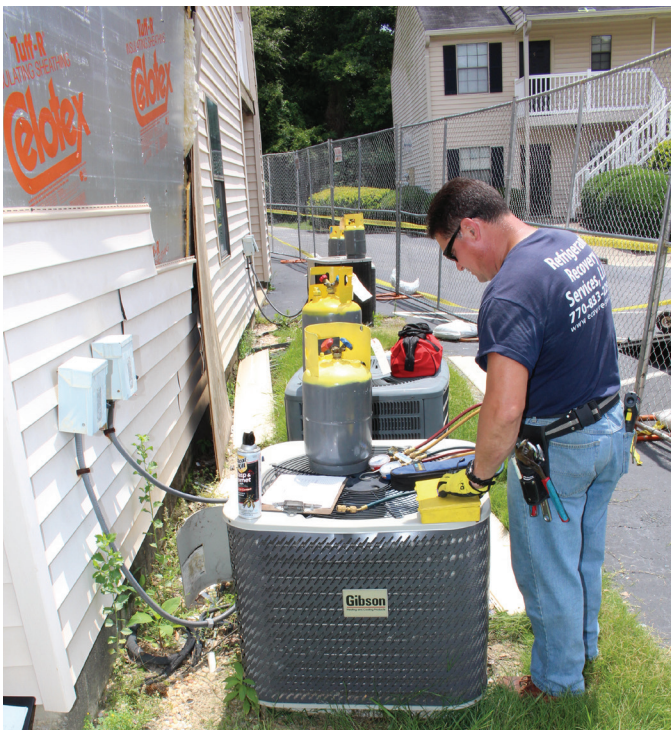
Figure 4 Outdoor split system heat pump unit.
